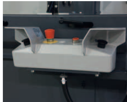
Two-handed operation instead of protection cover.
